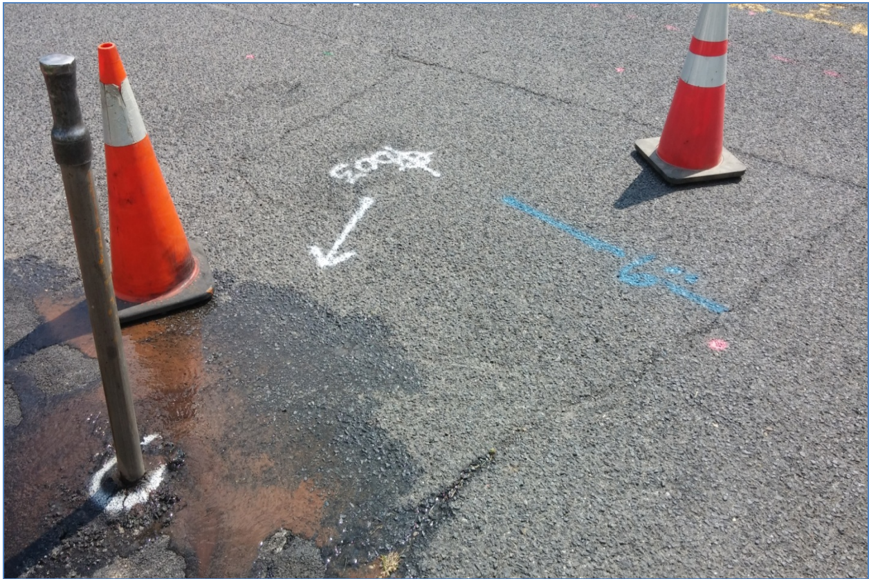
Photograph 1 - Water Line Strike
